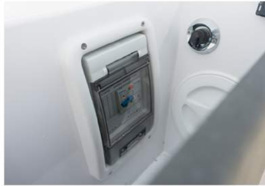
Shore power 230v with 20Ah charger
