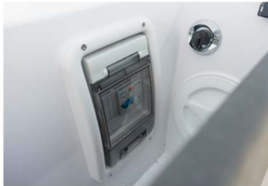
Shore power 230v with 20Ah charger
